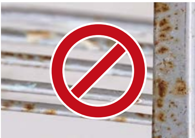
Rust and corrosion-free Save on cost of repair and replacement
